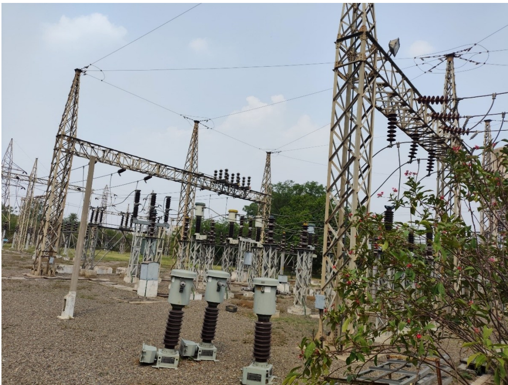
Figure 3:PSPCL Sub Station Patiala
